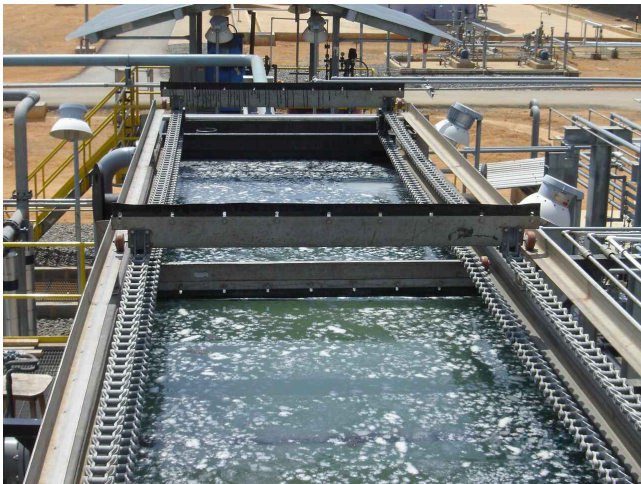
DAF with mechanical sludge scraper
